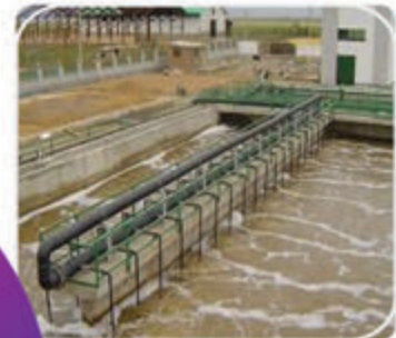
Urban Wastewater Treatment Sewage
